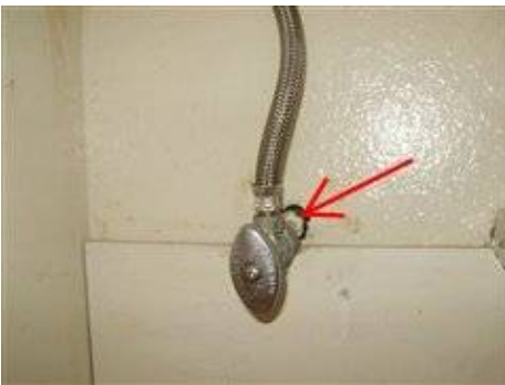
Photo 9 Gaps around undersink Shutoff Valve in Bathroom.
